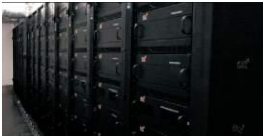
A123 2 MW Li Battery Array
